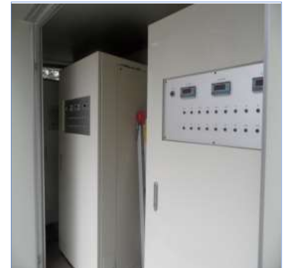
Load Bank (460V/100A)
